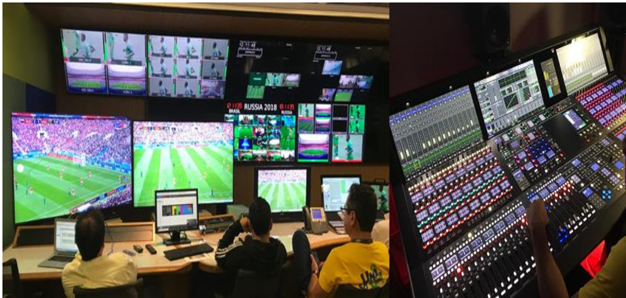
Figure 3 – CTRL 2 Control Room
