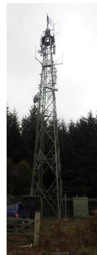
Figure 7 – Clun Transmitter Site
